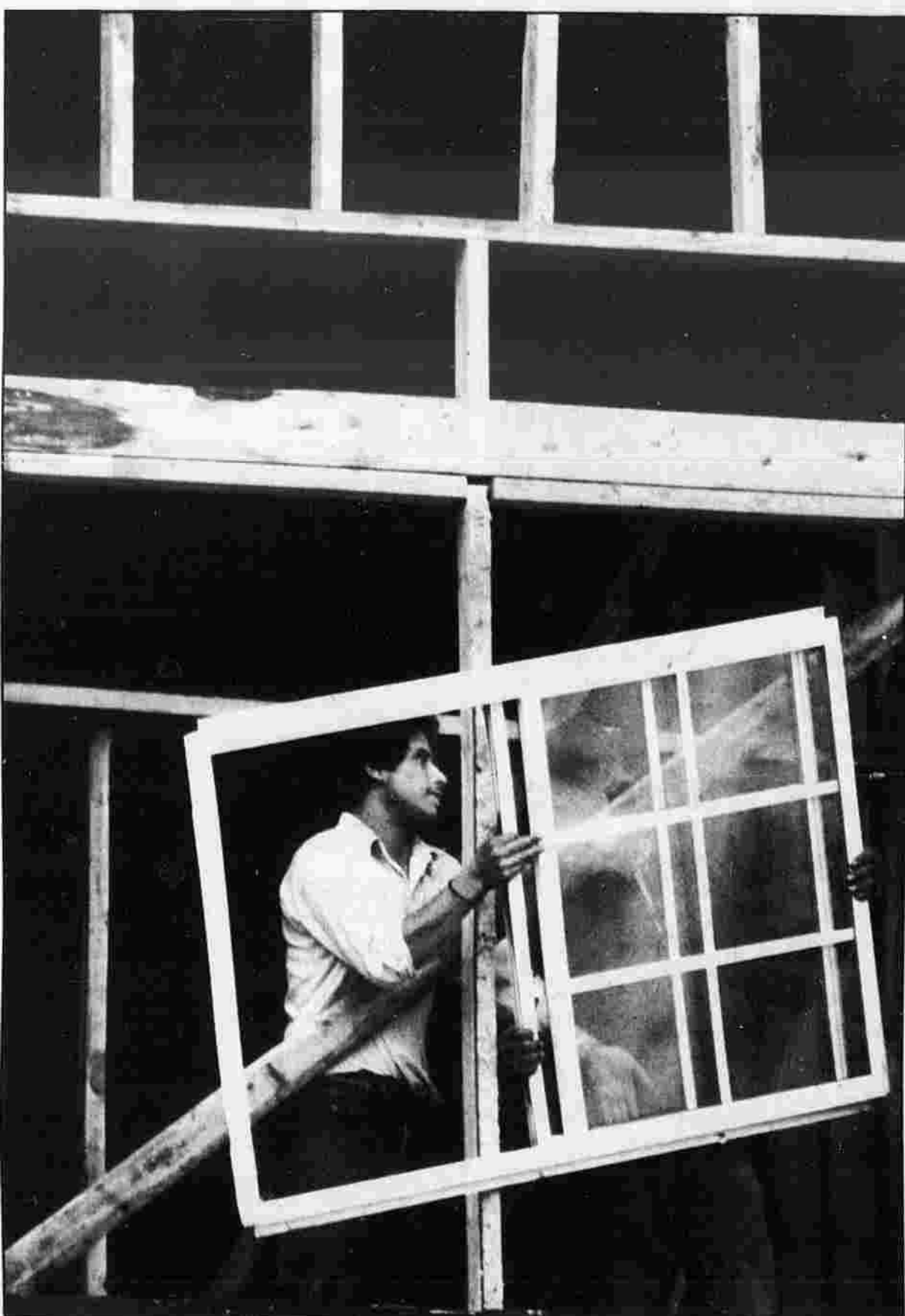
WINDOW WORK — David Martinez of Middletown, a carpenter employed by Franco Inc. of Glastonbury, installs windows at the Town Pavilions on Buckland Hills Road.
